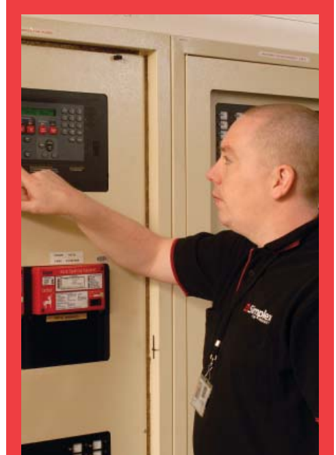
Simplex 4100U system, installed and operating in Crown Melbourne Limited
